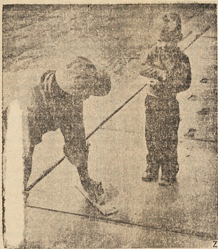
TROUBLE AFOOT — This little tyke is in a sticky predicament. While trying to cement a friendship with the workman who has just painstakingly finished the sidewalk, the chap really put his foot in it — but things were smoothed over in the end.
