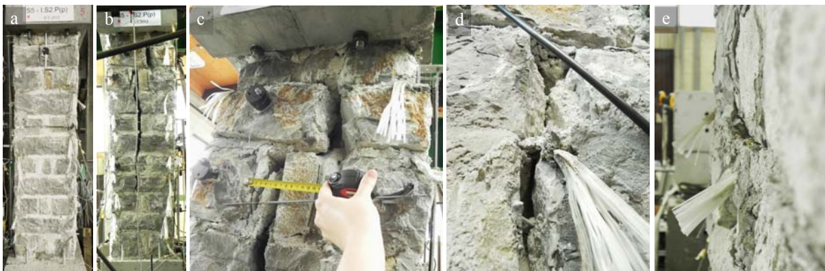
Figure 5.16: Leaf separation with toe-crushing (a-c), damage of the transversal connections (d, e) of the wall after test S5 - I.S2.P(p) Slika 5.16: Razpoka (vrzel) med slojema ter zdrobljena peta (a-c), poškodovanost prečnih povezav (d, e) zidu po testu S5 - I.S2.P(p)
