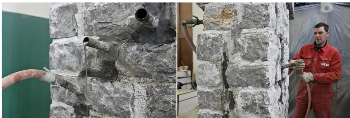
Figure 4.13: Leakage of the grout from a higher tube (left) and from a tube on the other side of the wall (right) (photos Željko Stevanić for UL FGG)
