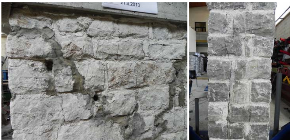
Figure 5.2: Damage pattern after failure attained at test T1 - I(n) Slika 5.2: Poškodovanost zidu po testu T1 - I(n)
