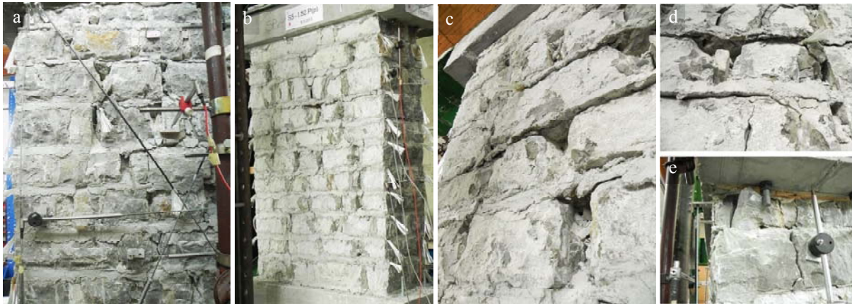
Figure 5.15: Crack pattern on the wall (a, b) with cord detachment (c, d) and toe crushing (e) after test S5 - I.S2.P(p) Slika 5.15: Razpokanost zidu (a, b) z odstopanjem vrvice (c, d) in zdrobljeno peto (e) po testu S5 - I.S2.P(p)
