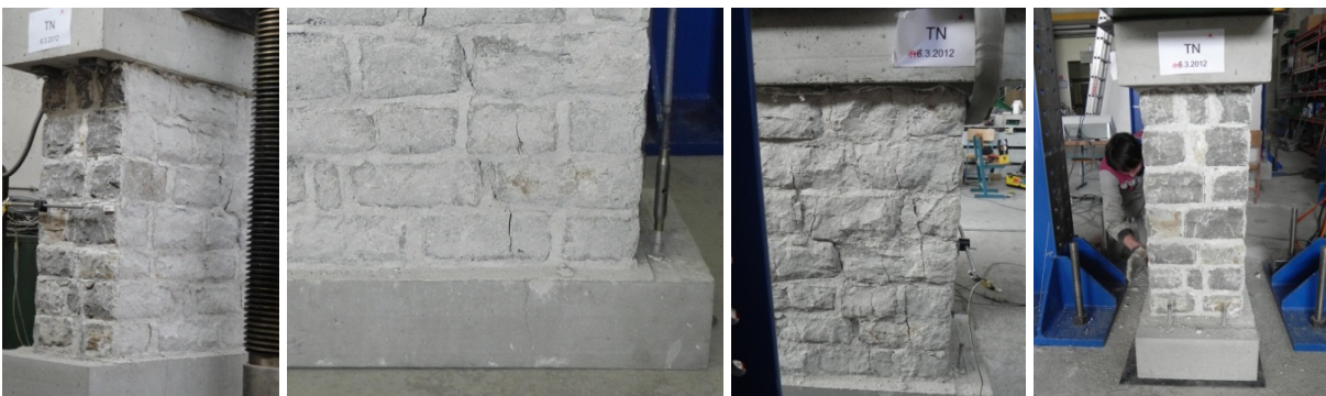
Figure 3.12: Damage on the walette without through stones due to non-uniform load distribution under hydraulic jack of 5000 kN capacity after the 1 st test (TN-1, left two) and after the 2 nd test under 2500 kN jack (TN-2, right two) Slika 3.12: Poškodbe na nepovezanem zidku zaradi neenakomerne porazdelitve sil pri 1. testu s 5000 kN batom (TN-1, levi dve sliki) ter po 2. testu z 2500 kN batom (TN-2, desni dve)
