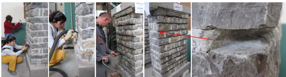
Figure 4.15: Process of emptying horizontal mortar joints: removal of mortar, vacuuming, water cleaning of emptied joints and wall with partially emptied joints
