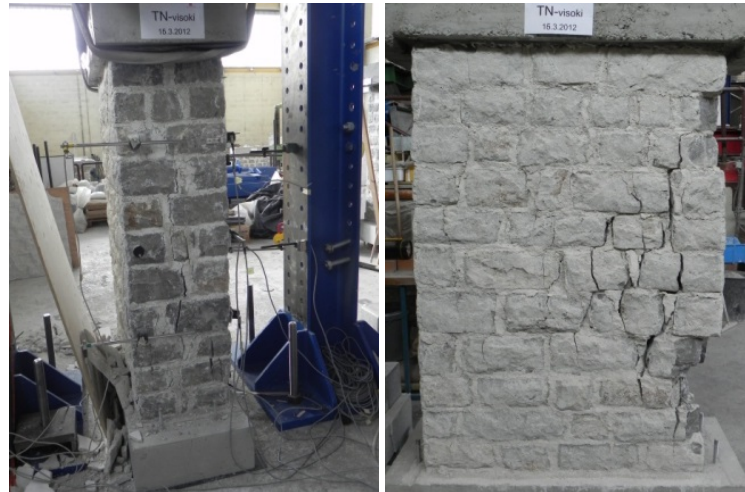
Figure 3.19: Damage of the wall without through stones after test TN-visoki Slika 3.19: Poškodbe na nepovezanem zidu po testu TN-visoki
