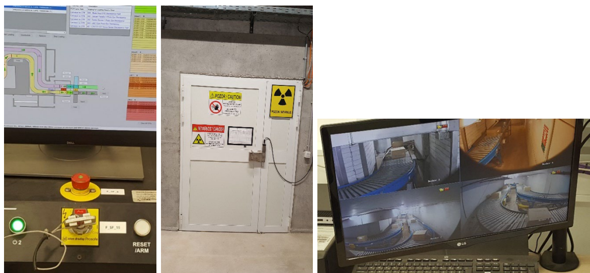
Figure 14: An operator controlling instruments with a master key used for entering into the bunker (left); the entrance to the bunker with a safety system (middle); video surveillance of the bunker interior (right) (Photo: the SNSA Inspection)
