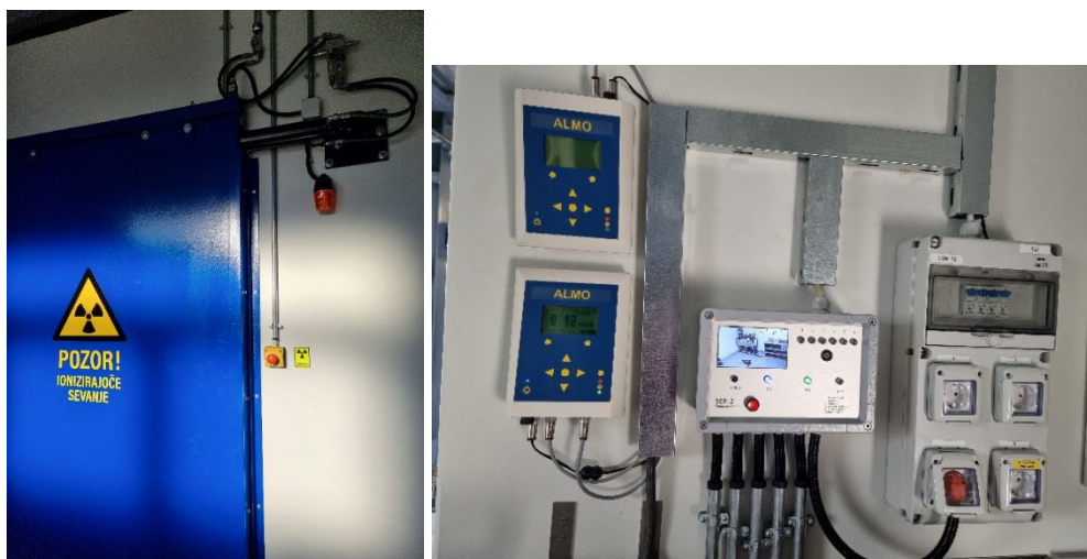
Figure 13: The entrance to the shielded enclosure dedicated to industrial radiography with a stop button and warning light (left); and controlling instruments used for carrying out and the control of industrial radiography (right) (Photo: industrial radiography operator)
