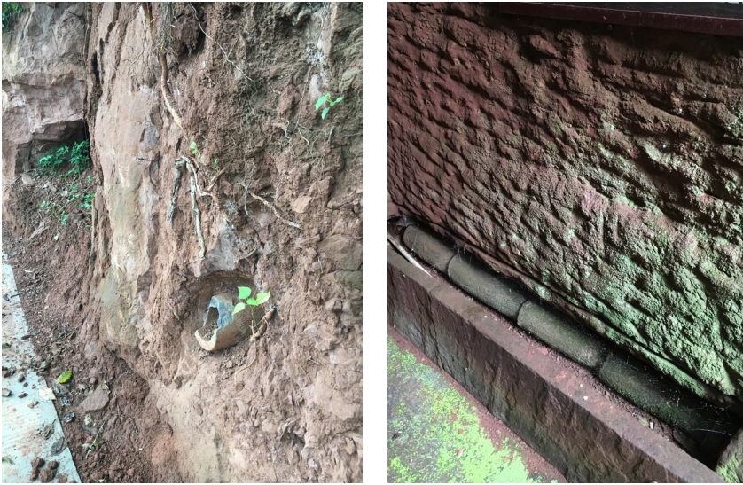
Figures 5a, 5b: Cliff tomb drainage pipes, Pengshan, Sichuan (Photos by Author).
