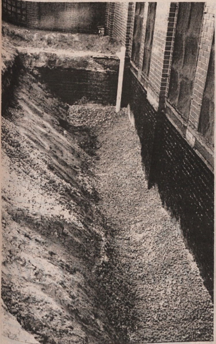
WORK NORMALLY NOT SEEN but necessary: Installation of drain tile, water proofing and gravel in back (north) side of St. Martin DePorres school building (formerly St. Vitus). This work seeks to divert and eliminate incoming water, primarily during heavy rain storms that occur in northeast Ohio during spring and fall seasons.
