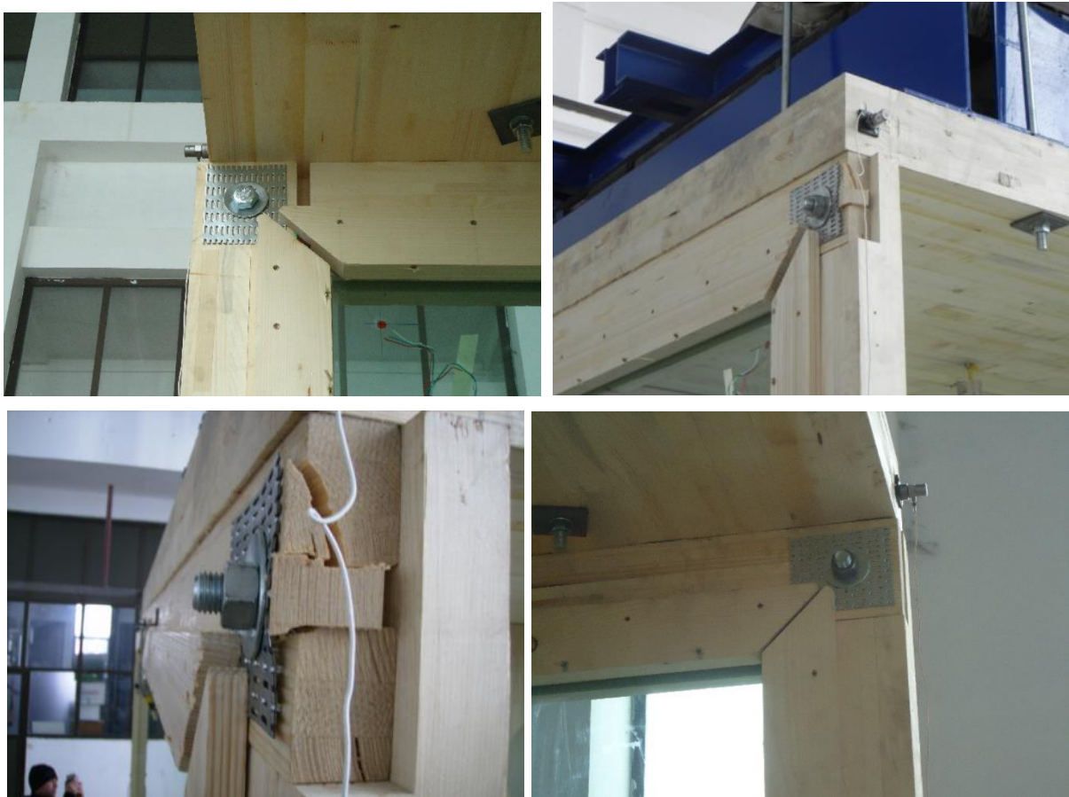
Slika 123: Identificirana poškodba preizkušanca v spoju lesenega okvirja pri a_g = 0,6g . Figure 123: Identified damage of specimen at the timber frame connection at the a_g = 0,6g .
