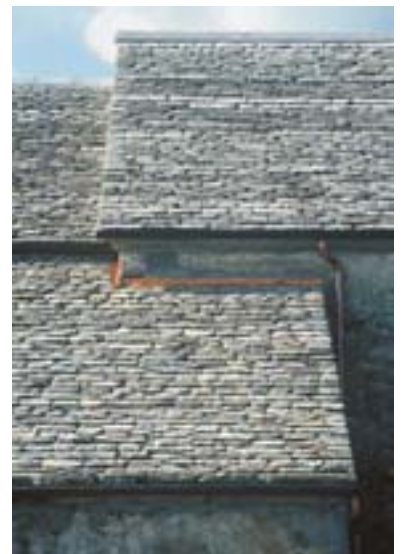
Slika 7: Obnovljena streha s kamnito kritino na cerkvi v Križu pri Sežani. Roof on the church in Križ, Sežana, renewed with stone roofing.
