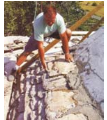
Slika 5: Polaganje skrl v malto pri obnovi cerkvene strehe v Križu pri Sežani. Laying slates in grout during renewal of the church roof in Križ, Sežana.
