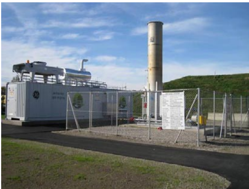
Figure 2: Small gas-operated power plants at the MSW landfill Dogoše [4].
